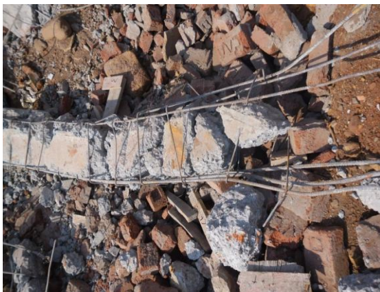
Fig 4 Destruction of concrete can be seen
