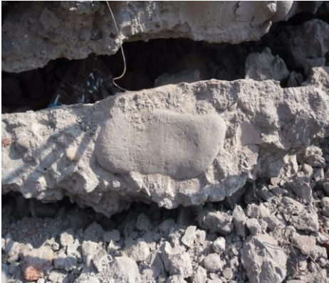
Fig 2 Presence of Cobbles In Concrete
