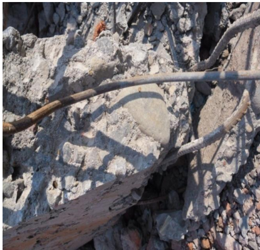
Fig 3 Presence of cobbles and boulders in concrete of beam
